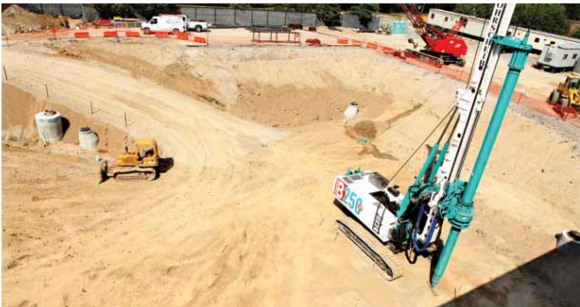
Mass excavation of the area where the new ME research complex will be is almost complete.
